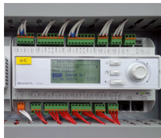
Controller box upgrade
